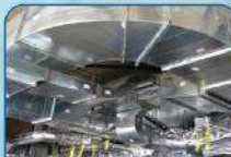
Laminar Ceiling with Air Diffusers
